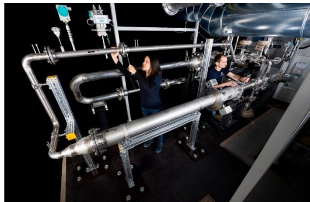
Figure 5: Set-up of the MGT test rig (without insulation), whole view
